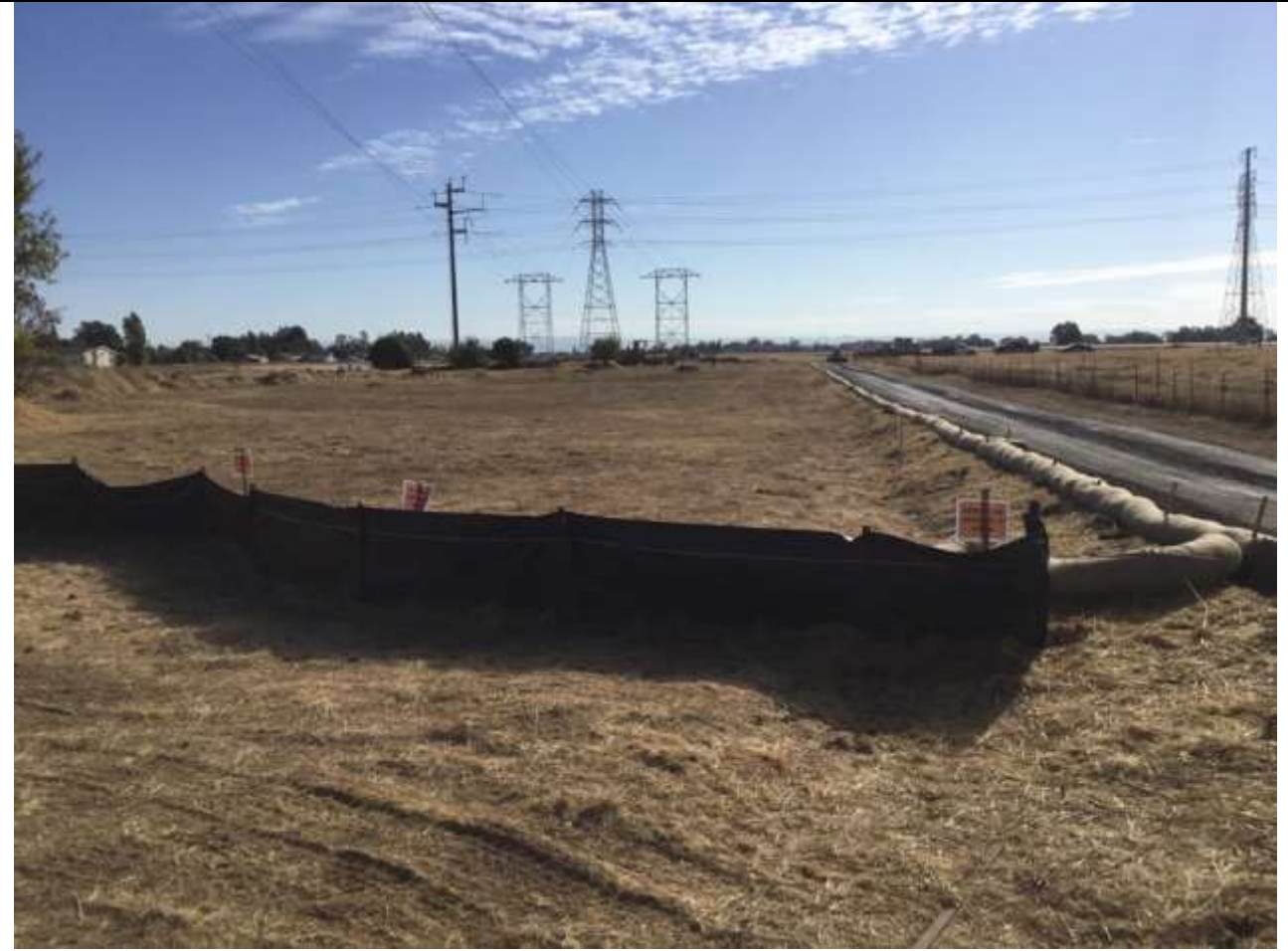
Photo 1: Exclusion fencing and installation of SWPPP BMPs are installed in accordance with APM BIO-6.
