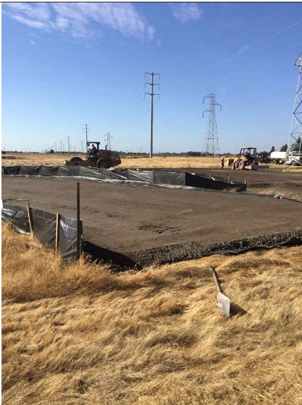
Photo 2: Completed winterization of landing/pull site for future reconductoring work at structure Palermo 0/1. Silt fencing has also been installed in accordance with SWPP BMPs.
