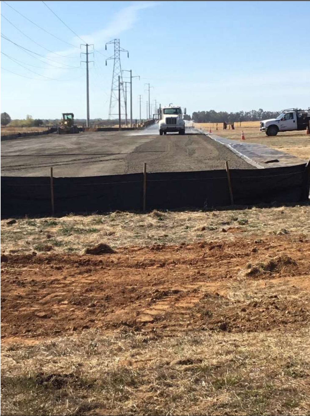
Photo 5: Water truck running to suppress dust during work at Pull Site 9/67 in accordance with APM AQ-1.
